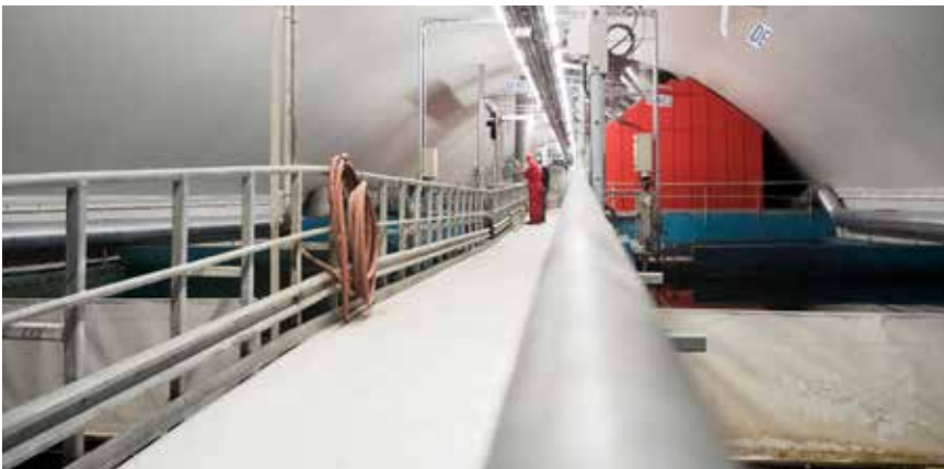
Due to climate conditions, all VEAS installations, including Filtralite nitrification and denitrification biofilters are situated inside the mountain
