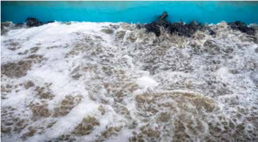
Filtralite biofilters are backwashed every day.
