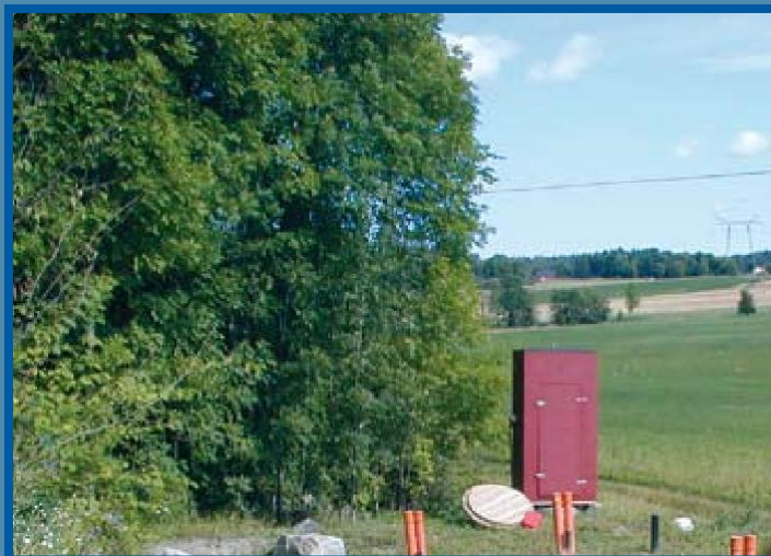
Photo 2 The pilot plant at Talby outside Stockholm. This plant treats sewage from Stockholm Vatten's office building at Bornsjön. The red shed contains sampling equipment used for taking daily and weekly samples.
