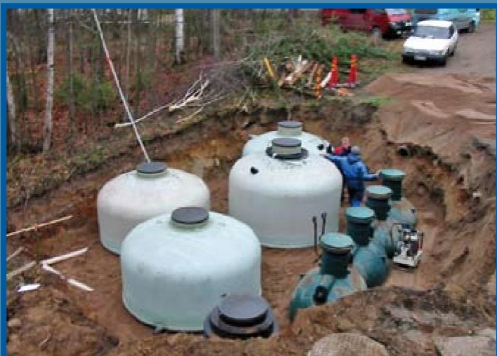
Photo 1 Showing the construction of a compact plant for two households in Kuusankoski, Finland. The picture shows the septic tank, two pre-filter tanks on the left and two tanks for phosphorus removal with Filtralite® P in the middle of the photo. The pre-filters are constructed with a recycling system.
