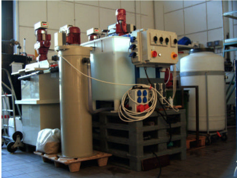
Fig. 2-3: Mixing tank (white, middle right), flocculant tank (ochre, middle left) and flocculation chambers (background left)
